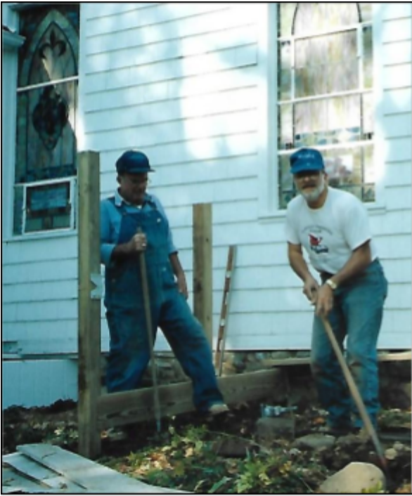
Lion Bob May (right), along with fellow Lions, building a ramp for handicapped persons at former Saddle River Valley Cultural Center in Upper Saddle River.
